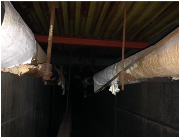
Piping with Asbestos
