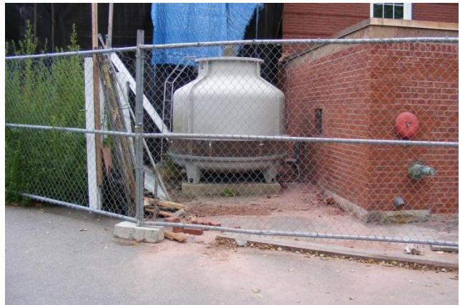
School Administration Building Mechanicals
