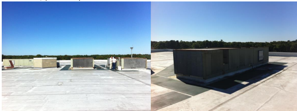
HVAC Roof Top Units ( RTU's ) at Barnstable High School and Barnstable Intermediate School
