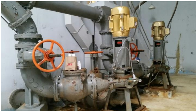
Freezer Road Pumps
