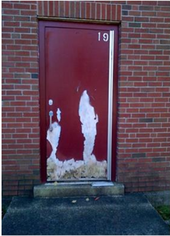
Hyannis West Elementary School Exterior/Interior Doors
