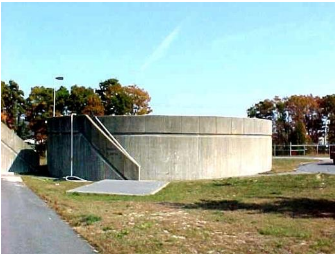
Water Pollution Control Facility – Clarifier
