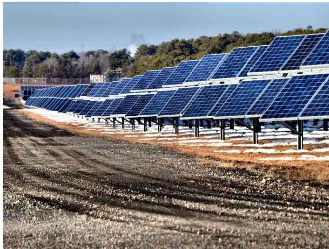
20-Acre Ground Mounted Solar Array Cape Cod Gateway Airport
